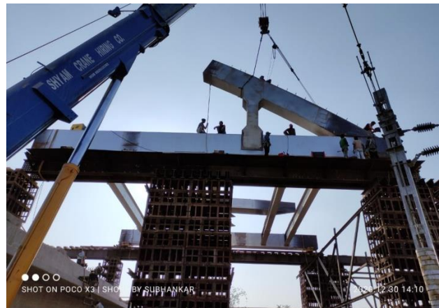
(b) Photo : Start of assembly of Bottom Beam, Top Chord, Hangers and Cross Girders
